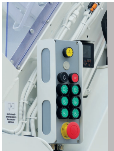
Operating controls at the rear
