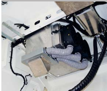
Cyclone filter unit
